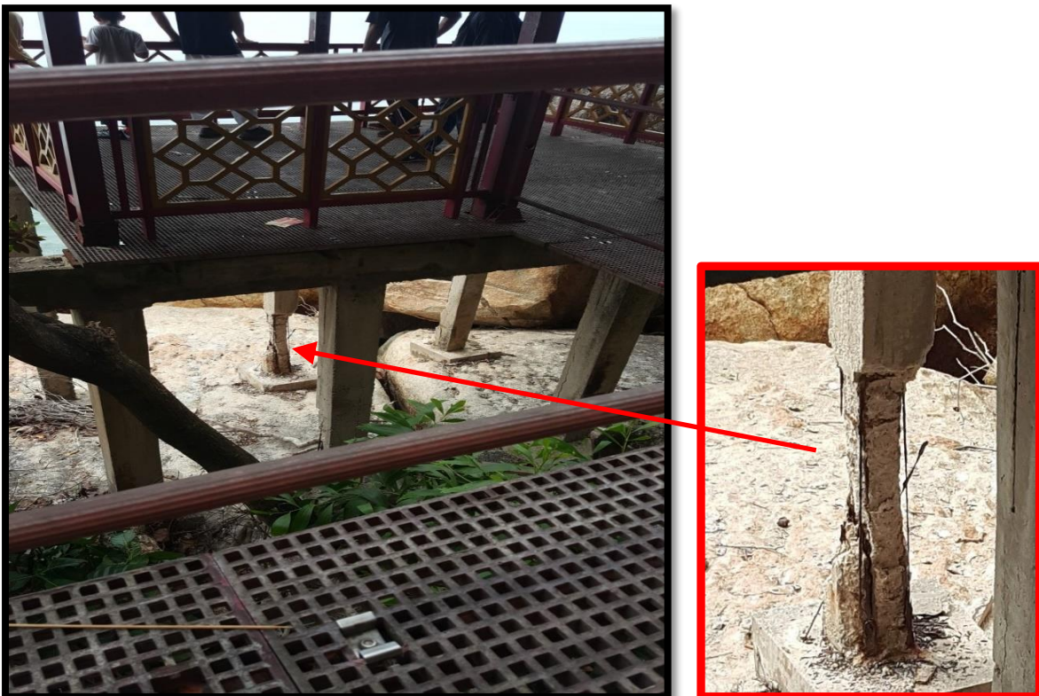
Figure 3: Badly Damaged Column with Considerably Total Loss of Rebar at a Coastal Building
