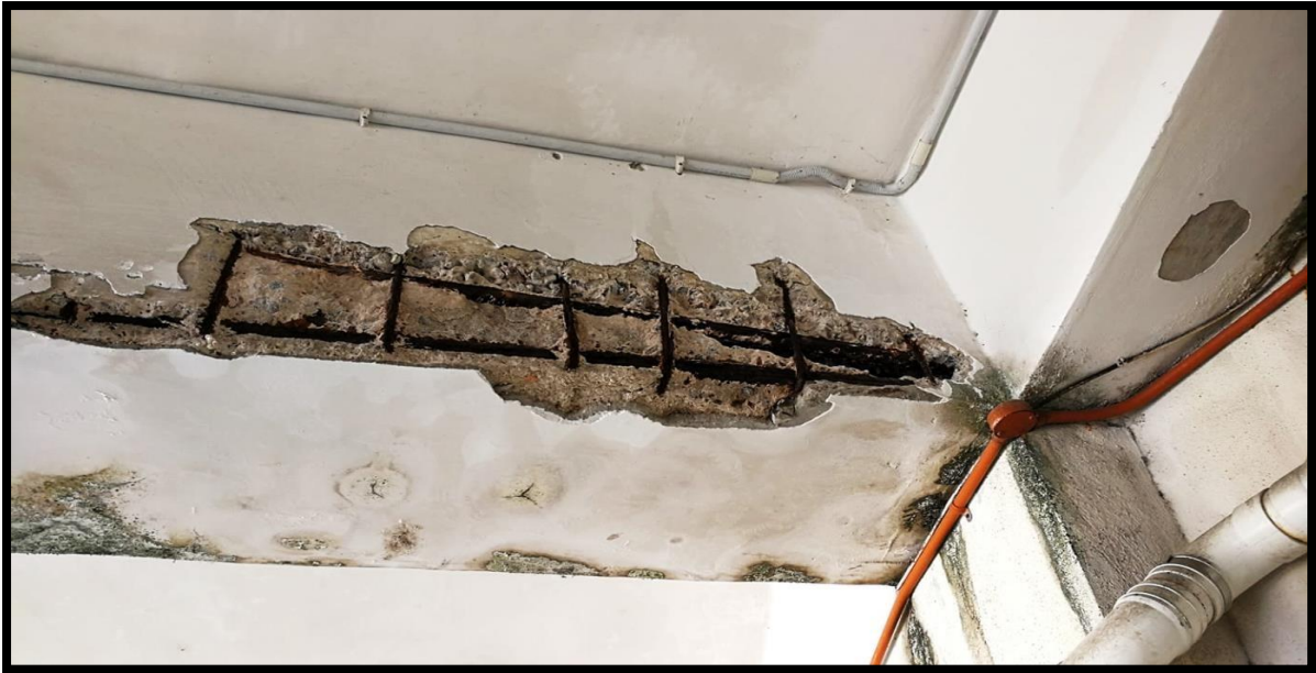
Figure 2: Concrete Spalling On a Beam Due To Moisture Intrusion
