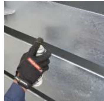
Figure 3: Inorganic zinc paint [7]
