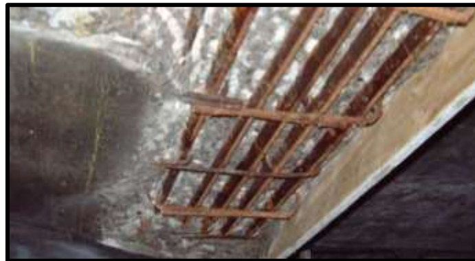
Figure 1: Corrosion of Steel Reinforcement in Concrete [2]
