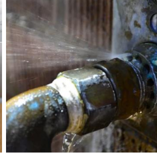
Figure 8: Old leaky pipe [10]
