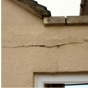
Figure 5: Cracks on wall [7]
