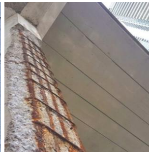
Figure 10: Corrosion of reinforced concrete structure [12]
