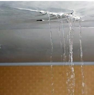
Rajah 7: Kebocoran bumbung [9]
